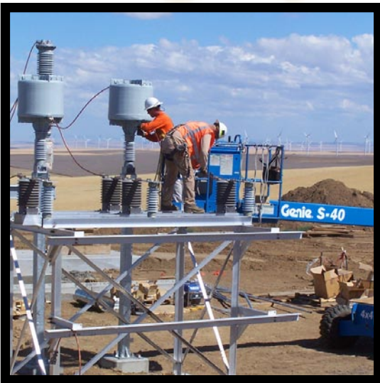
Electricians wiring switches and reactors at wind farm substation. Photo credit: John Demoss
