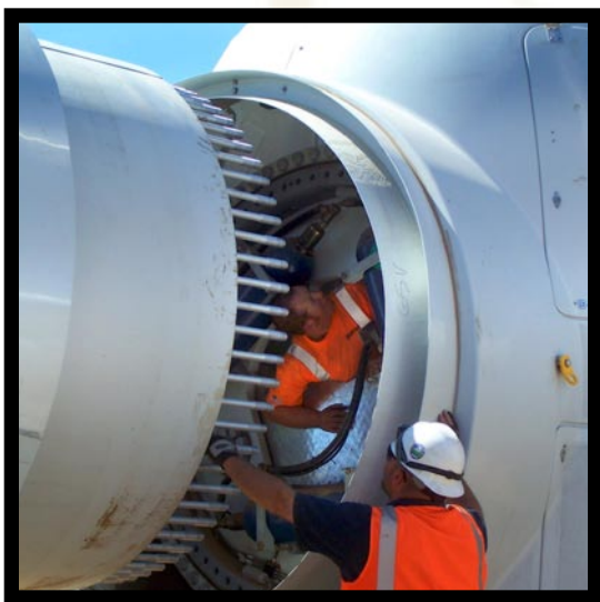
Wind Technicians aligning the bolt fit on wind turbine rotor assembly Photo credit: John Demoss
