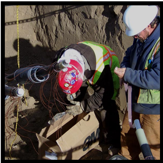
Technicians prepping wind turbine transmission cables for splice. Photo credit: John Demoss
